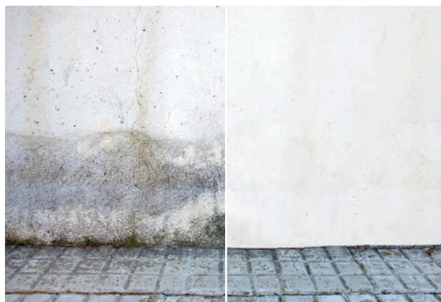
Cemento armato deteriorato Deteriorated reinforced concrete
